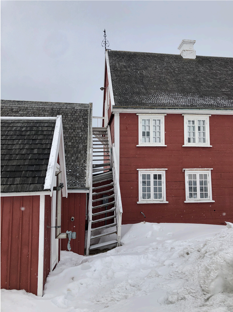
The High Arctic is considered particularly vulnerable to climate change. Climate adaptation of infrastructure and services is therefore particularly important in Greenland. The picture shows the effects of thawing permafrost on a building's stairs. Photo: Leneisja Jungsberg.
